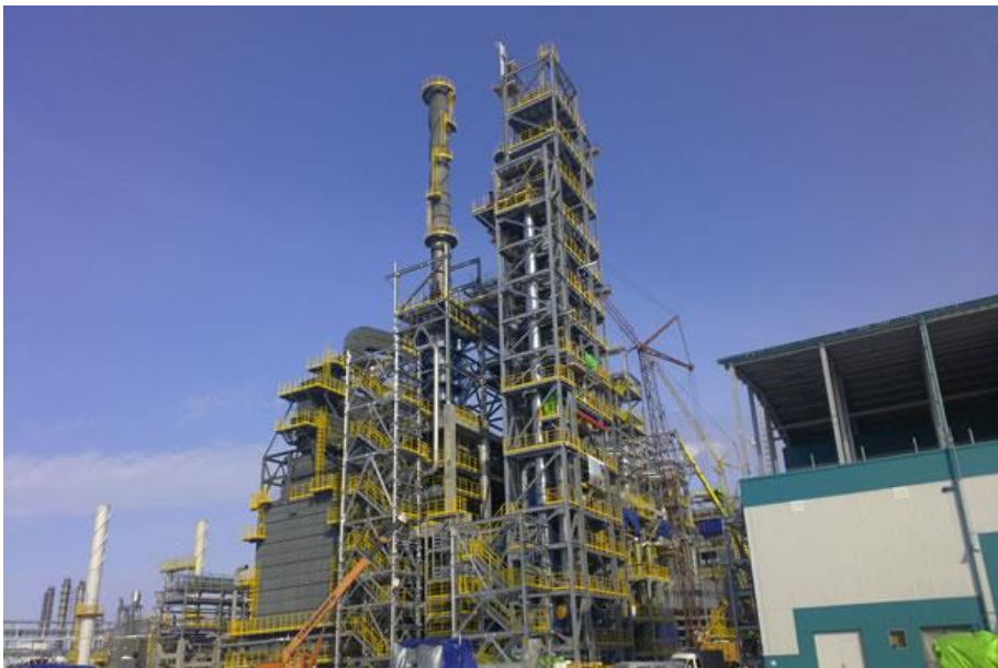
Figure 1 : Propane Dehydrogenation Unit (PDH) in Russia
